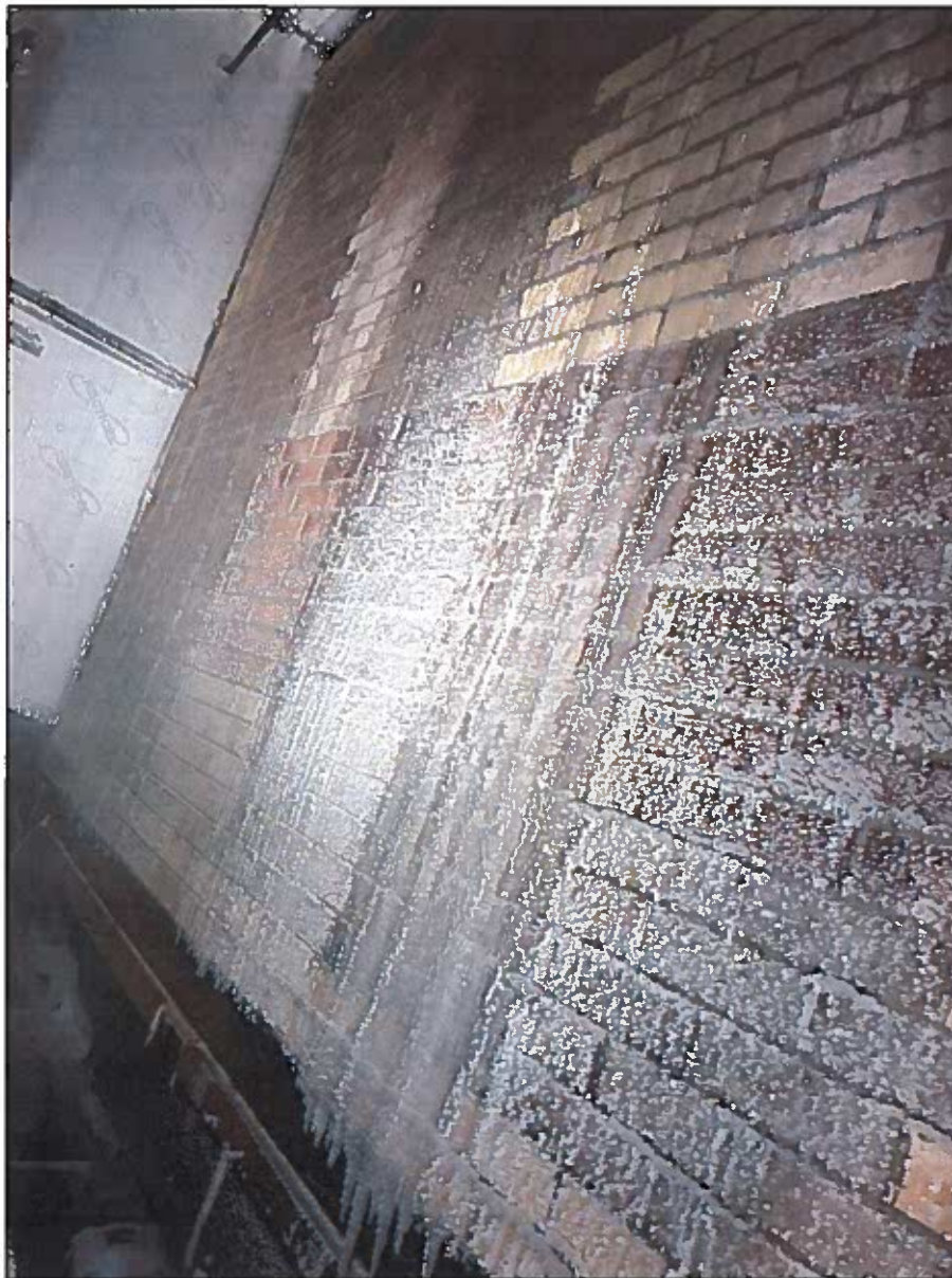
ICE BUILD UP ON FACE OF BRICKS SLIPS BEFORE THAWING
